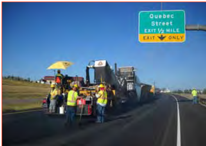
Crews place the final layer of asphalt on C-470 between I-25 and Santa Fe Drive following concrete repairs. The $808,000 project, which received $200,000 from the American Recovery & Reinvestment Act, also made improvements to the bike trail between I-25 and I-70 [Region 6].
