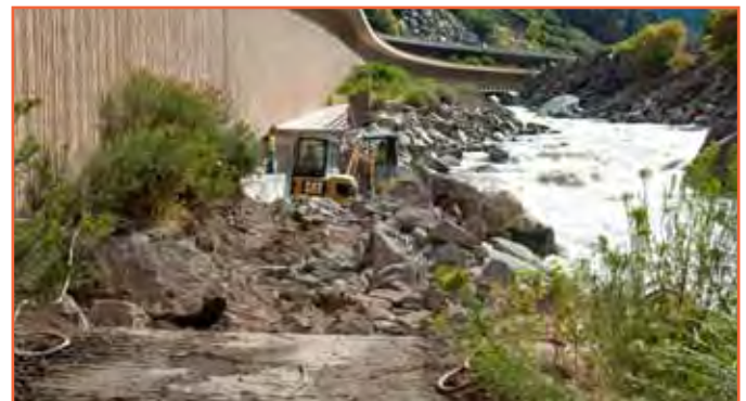
Emergency repairs of the I-70 Glenwood Canyon bike path following spring flooding included replacing 360 square yards of sidewalk on both on-ground and cantilevered sections. These complex repairs cost approximately $1.5 million, with assistance from the Transportation Commission's contingency fund. [Region 3]
