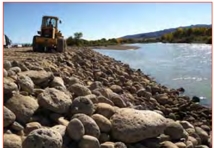
Emergency repairs were made along the Colorado River embankment along I-70 west of Fruita, with funding from the Transportation Commission [Region 3].
