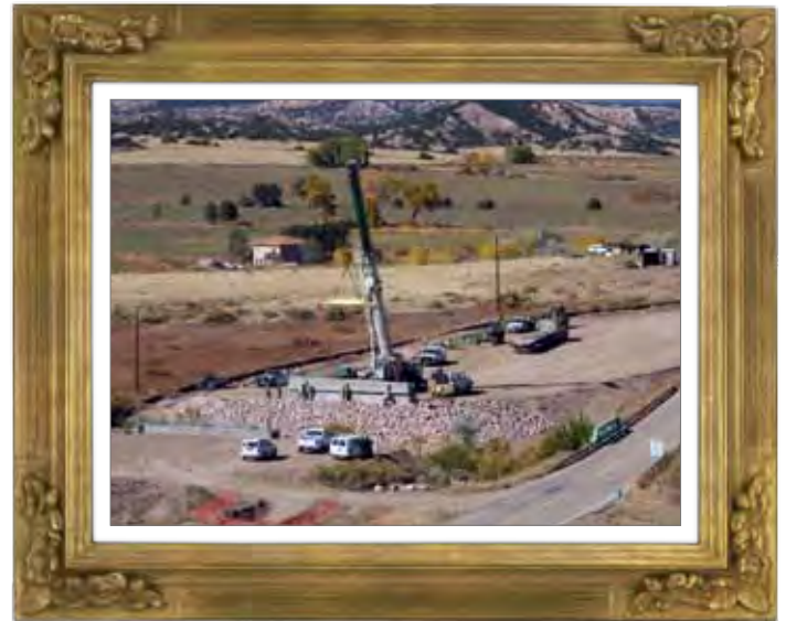
The First FASTER funded bridge project was at SH 69 over Turkey Creek in Huerfano County
