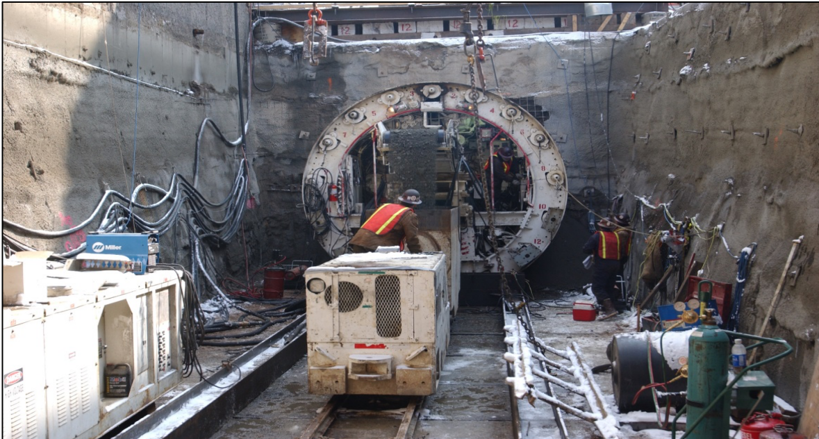
Drainage pipes on south I-25. While the Central 70 system won't be exactly the same, it is being built to handle a 100-year storm event.
