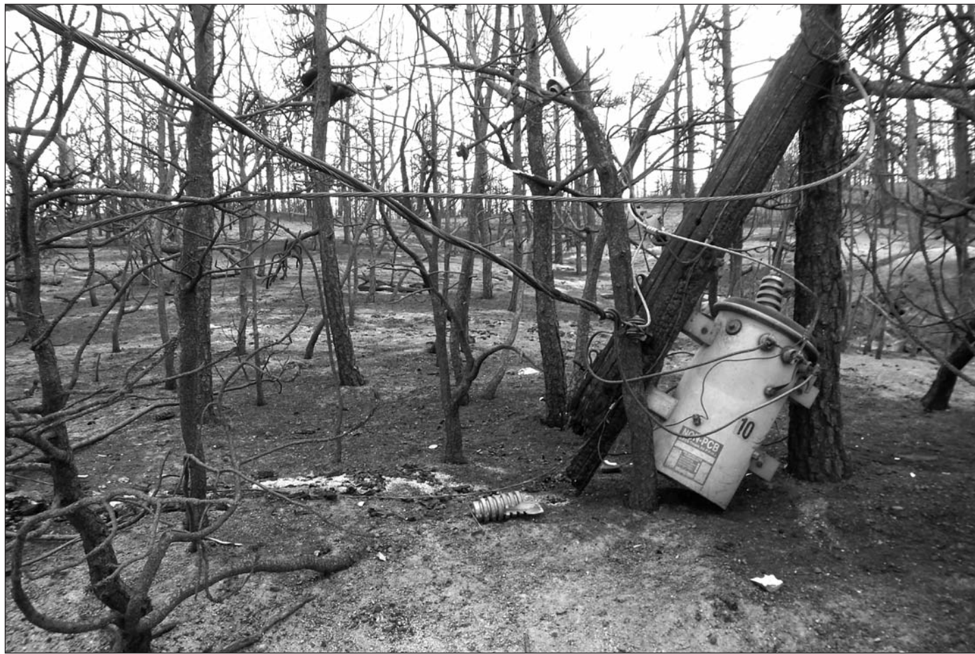
Fire damaged utility lines and equipment during this summer's Black Forest Fire near Colorado Springs. The PUC provides support on energy matters to the State Emergency Operations Center during wildfires and other disasters.
