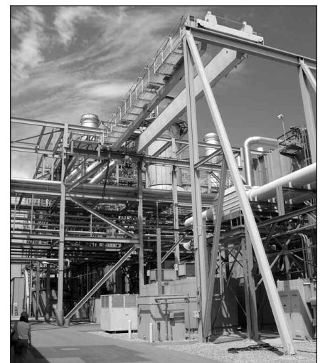
Fort St. Vrain Generating Station in Platteville.
