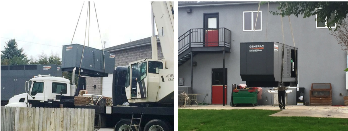
A crane lowers a backup generator funded under DR-4145 HMPG, at Station #2 for the Evans Fire Protection District Fire.
