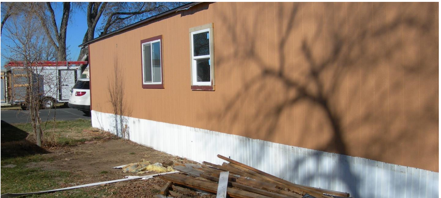
Christian Public Service provided services to rebuild the skirting on a mobile home for a family affected by the floods.
