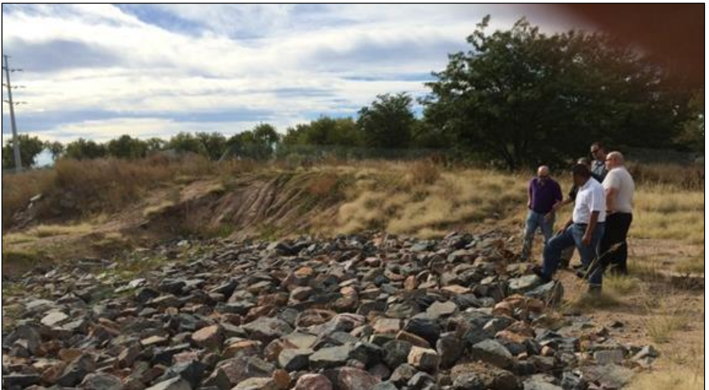
Evans berm inspection team at the field inspection of this NRCS project.
