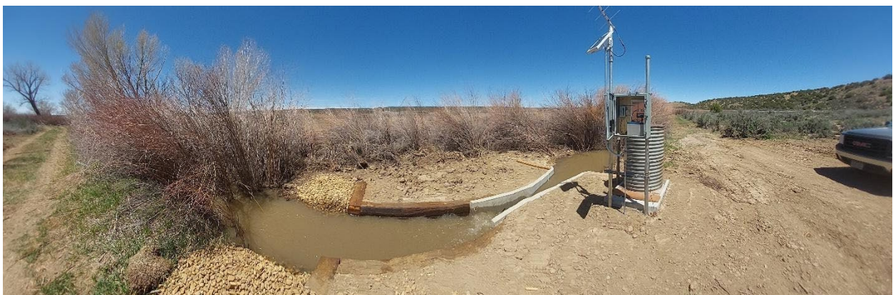
Figure 4: Completed new Pioneer Ditch Gauge.
