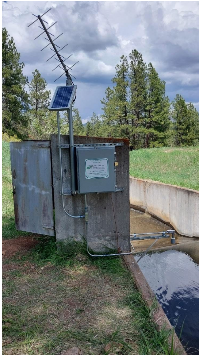
Figure 6: Jackson Parshall Flume to the West Mancos River
