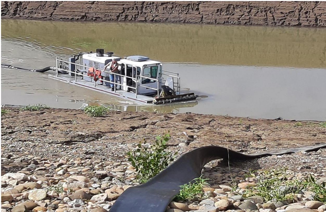
Figure 2 - Dredge used by Bureau of Reclamation to dredge canal at Great Cut Dike at McPhee Reservoir
