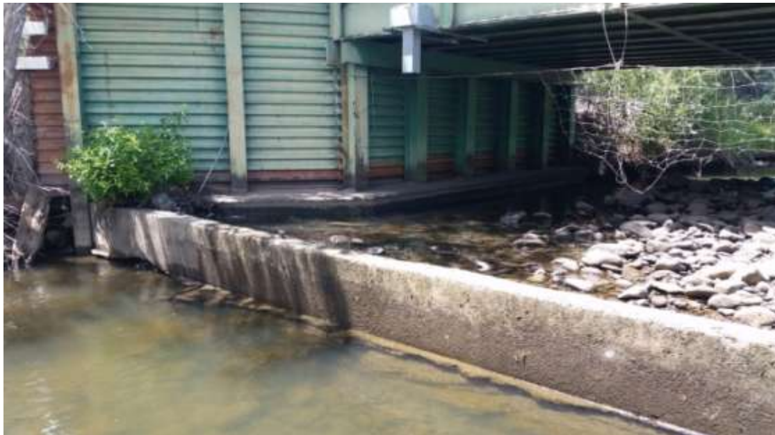
Figure 1: Down looking radar installed on CJ's Bridge on Mancos River
