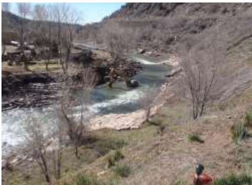
Construction of the City of Durango White Water Park (Recreational In-Channel Diversion)
