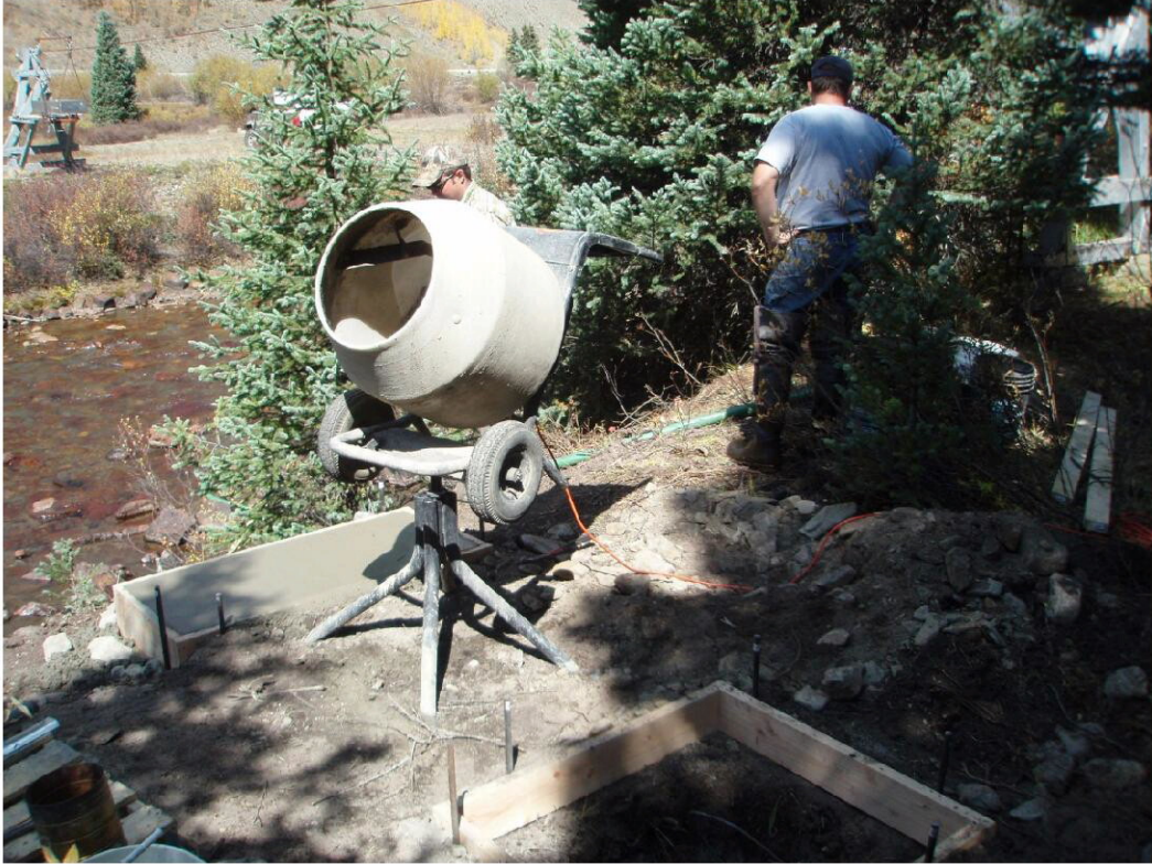
Picture taken at Animas River at Howardsville gaging station. Construction of unmanned cableway by Division 7 hydrographers and water commissioners.
