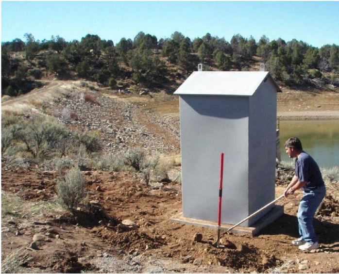
Brian Boughton installing a Sutron Accu-Bubbler at Red Mesa Ward Reservoir in October 2007
