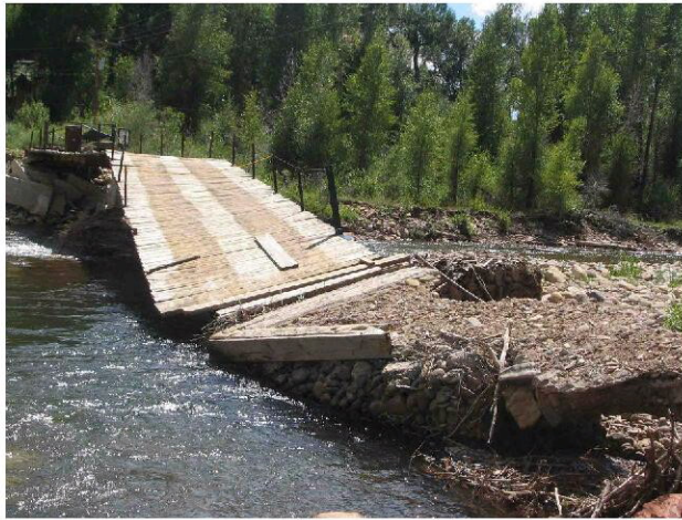
Bridge washed out on the East Fork of the Dolores River
