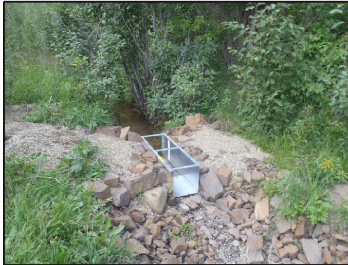
Nu-Way Flumes installed in ditches located within the Elk River Basin
