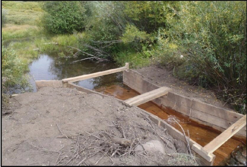
Picture of a newly installed wooden flume after ditch was shut off during Elk River administration due to not having a measuring device
