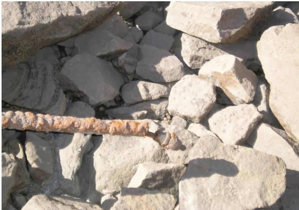
Corroded Conduit at Pearl Lake
