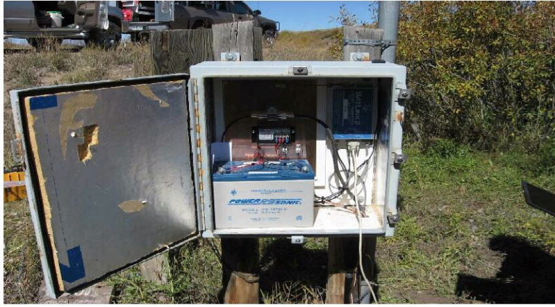
HDR DCP Installed at the Illinois River near Rand Gage Station
