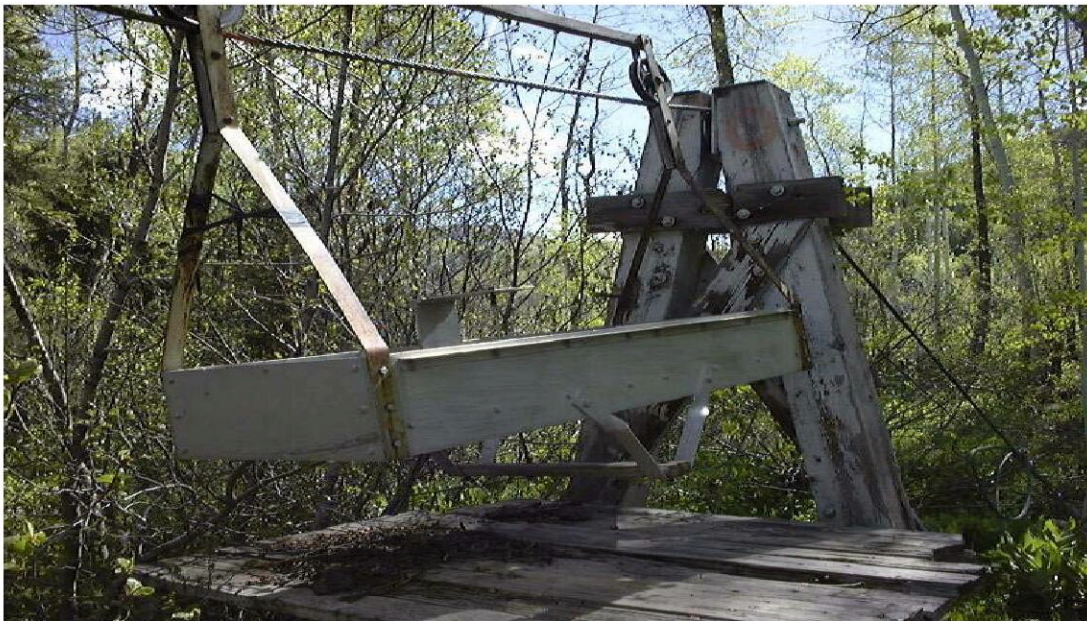
Condemned Cableway at the Walton Creek Gage Station
