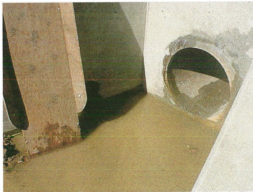
The downstream end of the new steel pipe during the grouting. This end was completely sealed with a new hydraulically efficient headwall.
