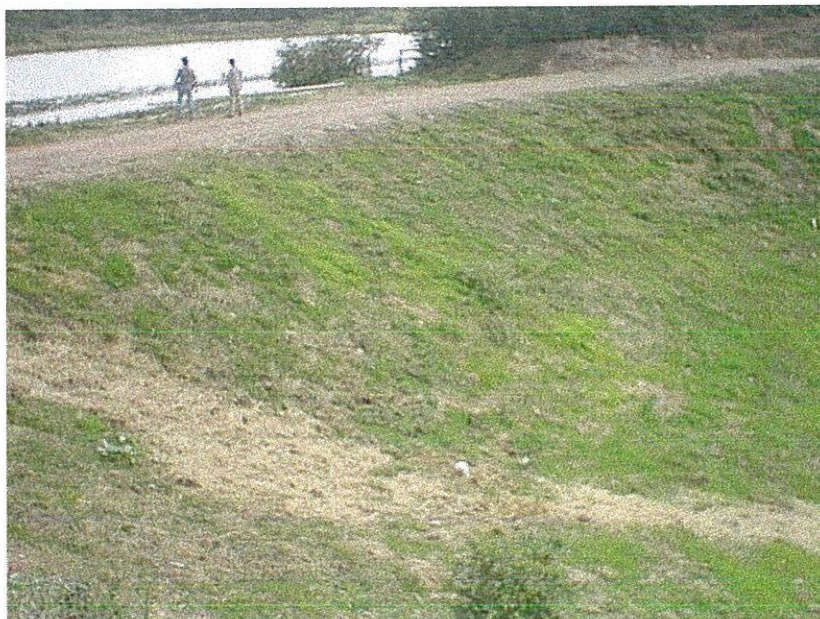
The completed downstream slope of the Thomas Reservoir Dam on August 27, 1999. This slope used to be covered with large trees, was very steep, and exhibited seepage.
