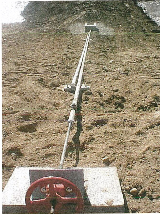
The new outlet stem and intake structure for Bumgarner Reservoir.
