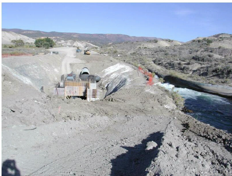
South Canal Hydroelectric Project 2013 – 4 Megawatts
