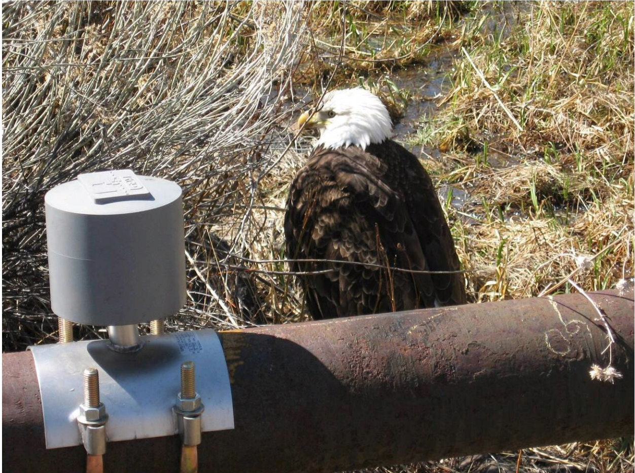
The eagle eyes in Division III inspecting a new well meter.
