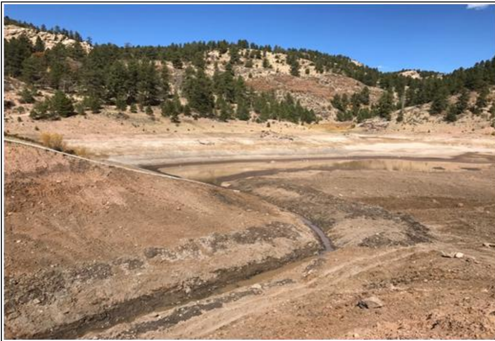
Figure 5: Breach of Riss Complete
