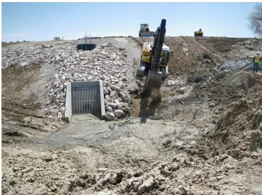
Martin Lake Dam – completing the upstream toe near the new outlet headwall.
