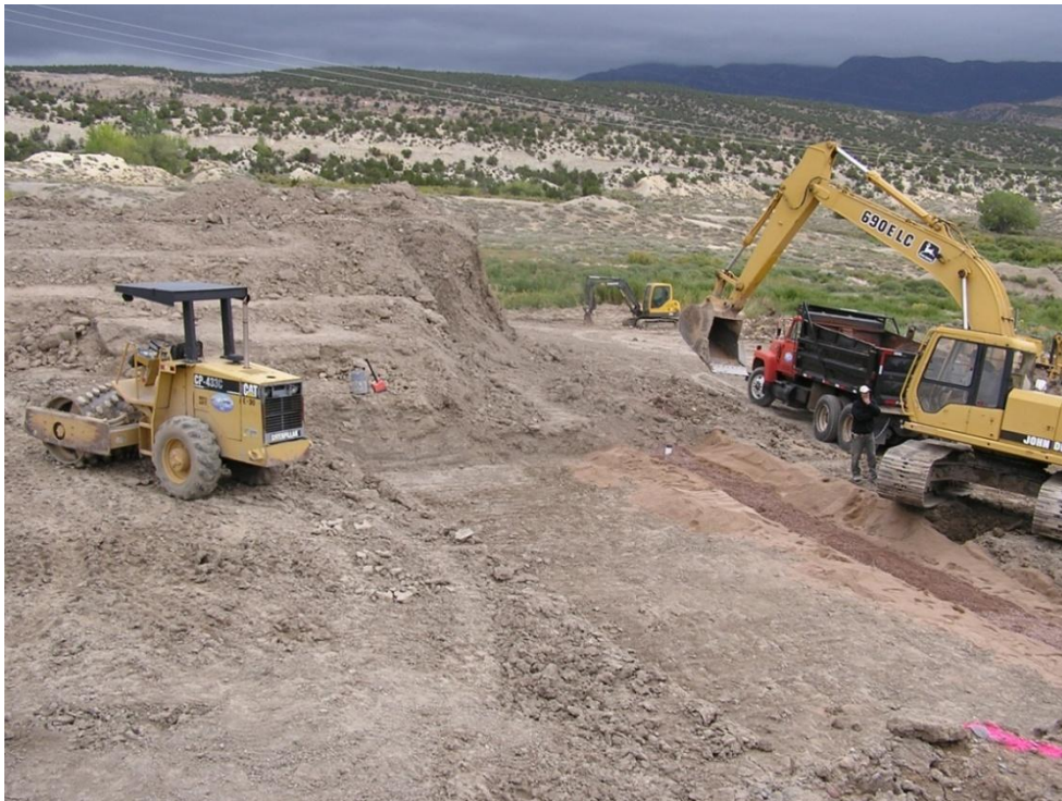
Repairs to the Park Center #5 dam after a seepage pipe developed in the dam. The embankment was breached in the area where seepage developed. Cracks were excavated and the dam was reconstructed with a filter drain in that breach.
