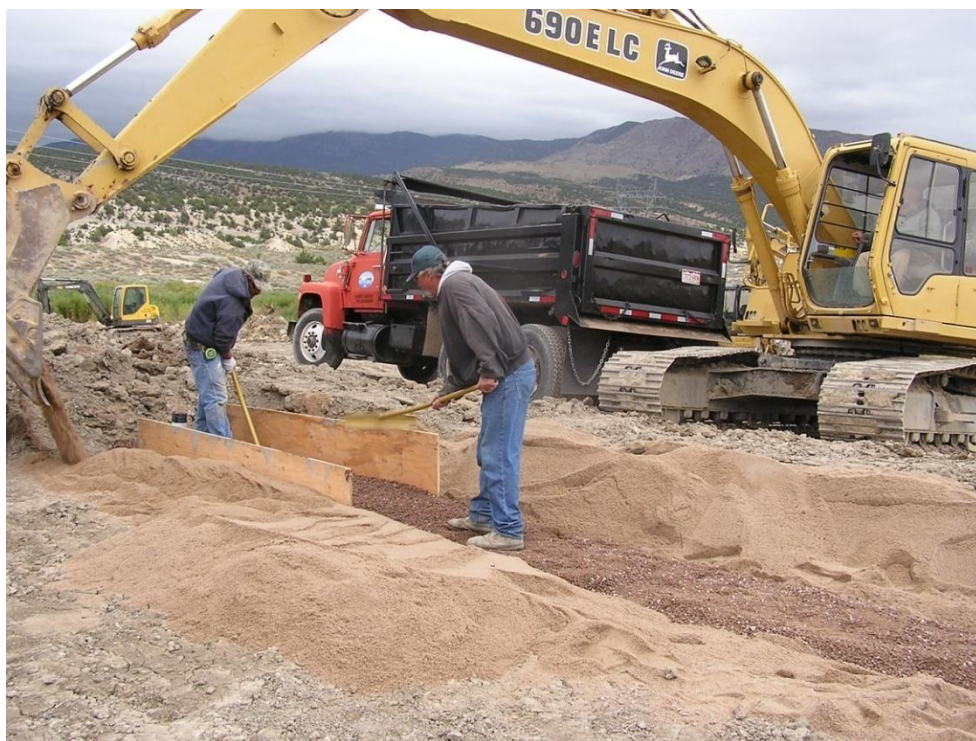
Installation of a two stage filter at the downstream toe of Park Center #5 dam.
