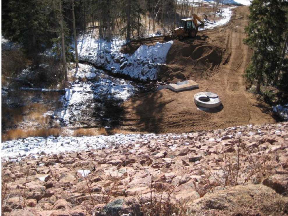
Photo No. 3 – View looking down on the new outlet works discharge structure at the toe of Palmer Lake No. 5 Dam.
