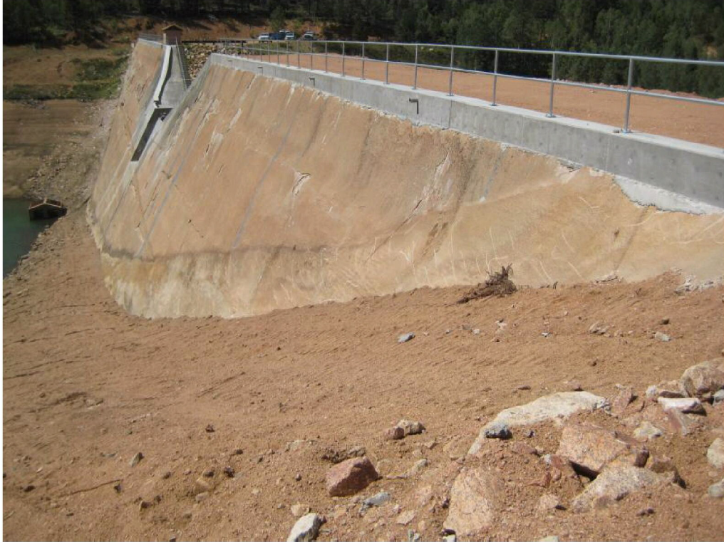
Photo No. 1 – Parapet wall completion and cleaning of upstream face in preparation for Carpi geomembrane lining installation at Big Tooth Dam in the mountains above Manitou Springs.
