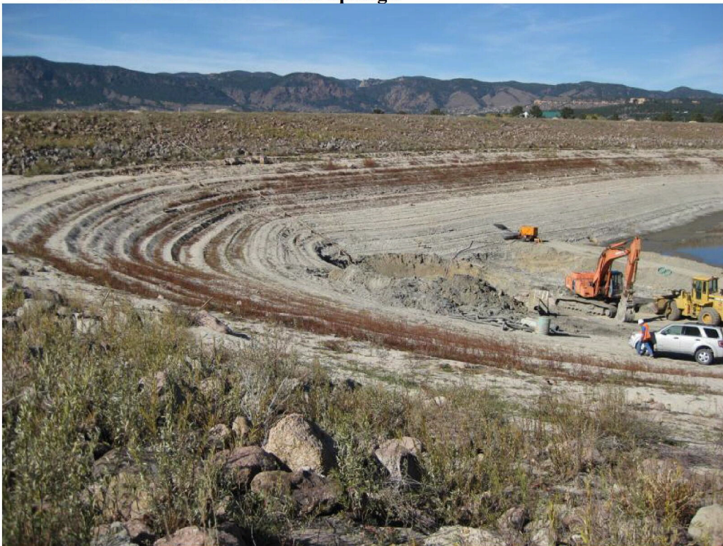
Photo No. 2 – Drained reservoir and work progressing on the outlet works rehabilitation project at Woodmoor Lake Dam.
