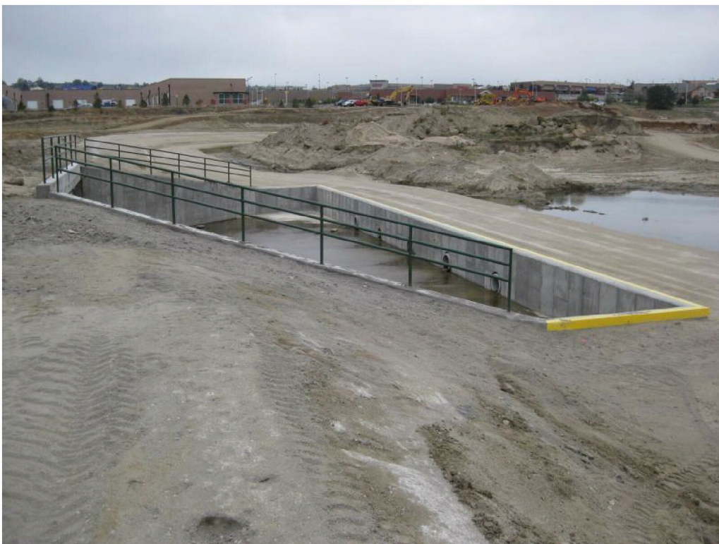
Photo No. 4 – Inlet area on the upstream face of the new Sand Creek Detention Dam No. 2 in Colorado Springs.
