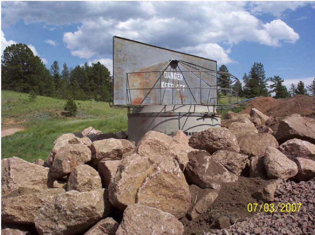
Photo No. 3 – Overflow structure repairs at Jordan No. 1 dam near Cripple Creek.
