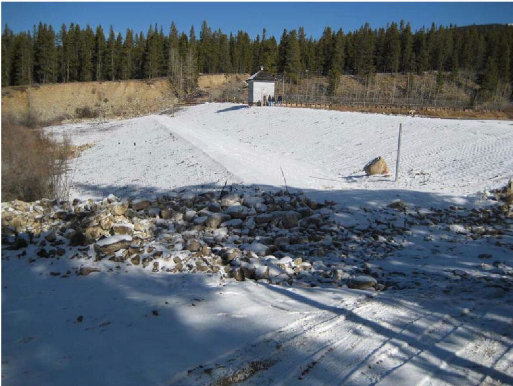
Photo No. 2 – Stability berm and toe drain installation at Evan’s Gulch dam in Leadville.
