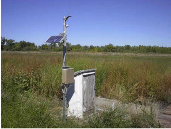
South Platte Flow Monitoring Project Telemetry at the South Reservation Ditch
