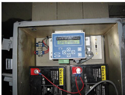
Stage Discharge Recorder
