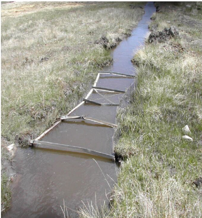
Poorly Installed Flume (Dist 23). Photo shown at Contractor Training in Sterling
