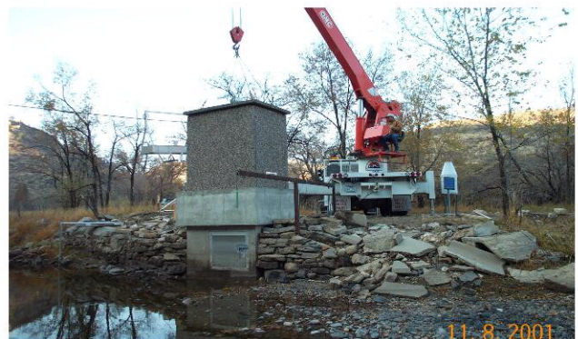
Poudre Canyon Gage After Raising For Flood Protection
