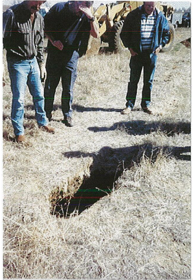
Sinkhole As Exposed After Truck Drove Over It
