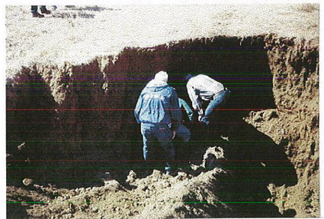
Inspection of Sinkhole After Opened Up By Backhoe
