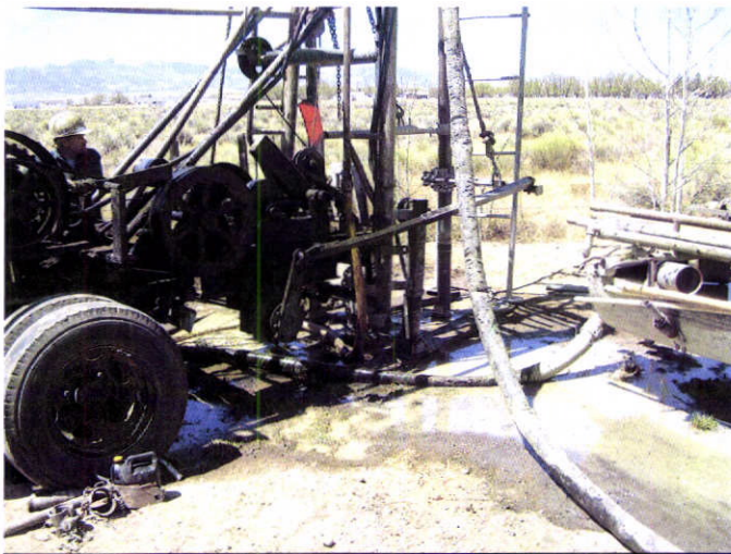
A unique old spudder drill rig drilling a well in the San Luis Valley.
