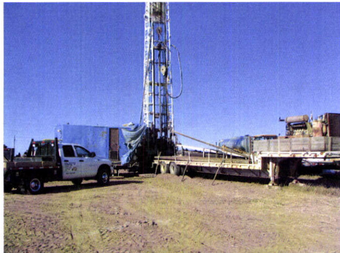
Drilling a domestic well in the Fox Hills formation near Keensburg, CO.
