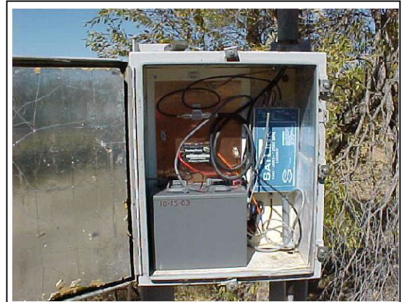
High Data Rate Installation at Smith Ranch
