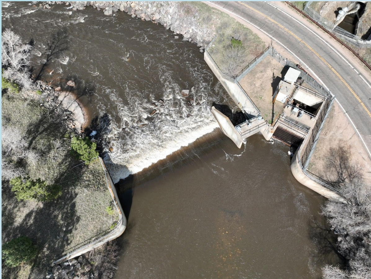
Munroe Diversion Structure, photo by David Bridge
