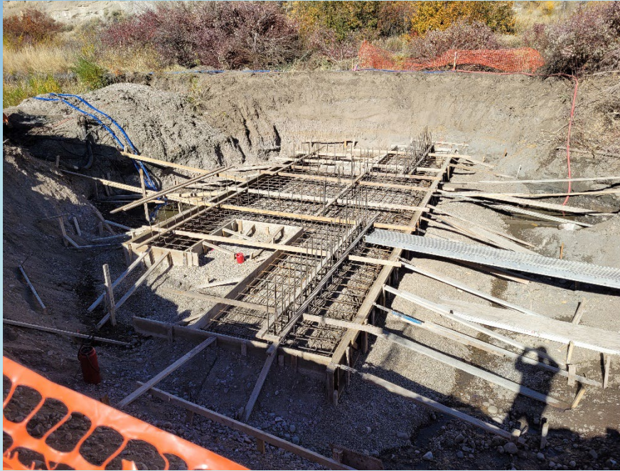
Gibraltar Ditch new headgate, photo by Brian Romig
