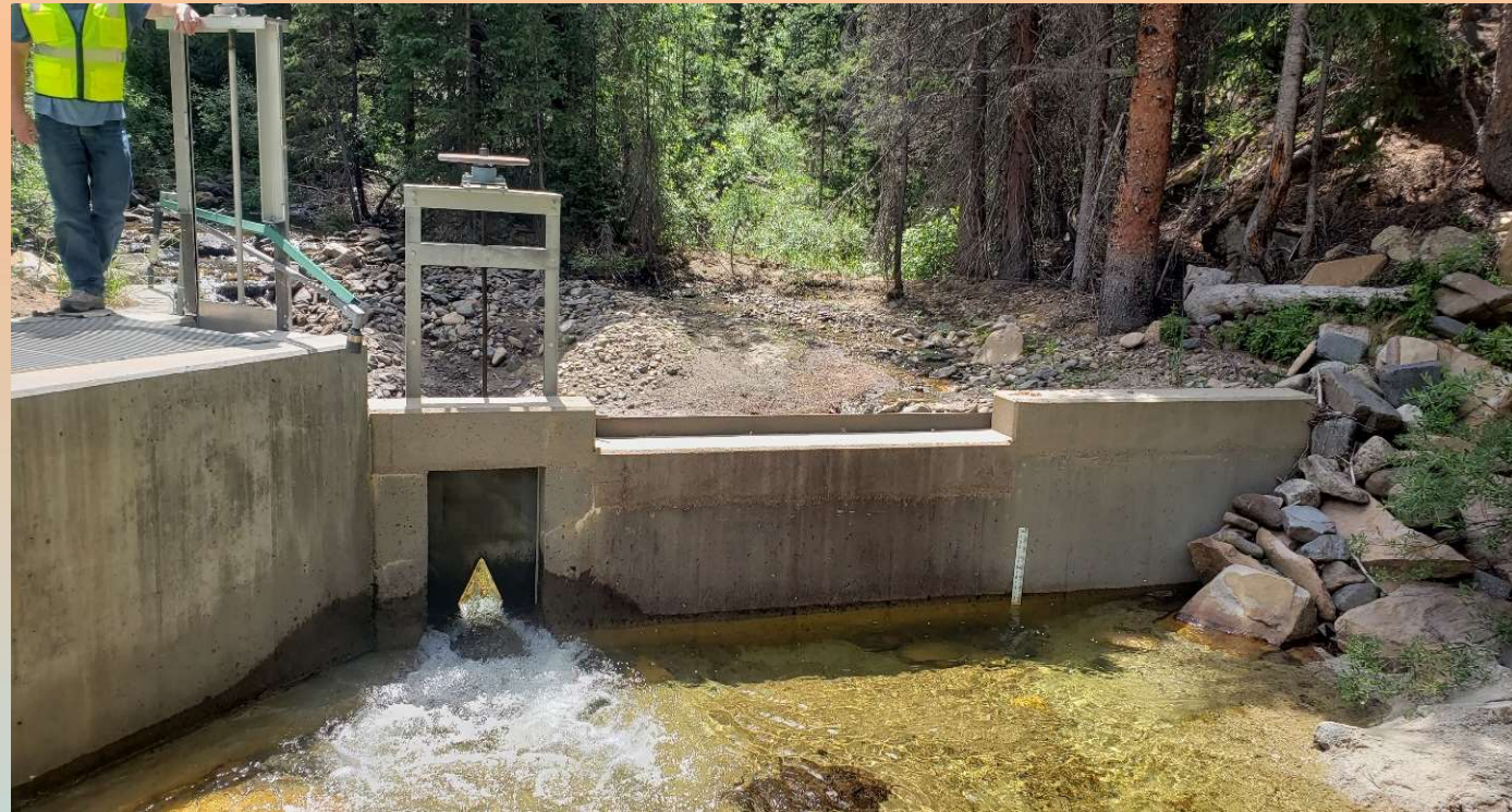
Diversion structure for the East Fork Pumping Plant. Photo by Jana Miller
