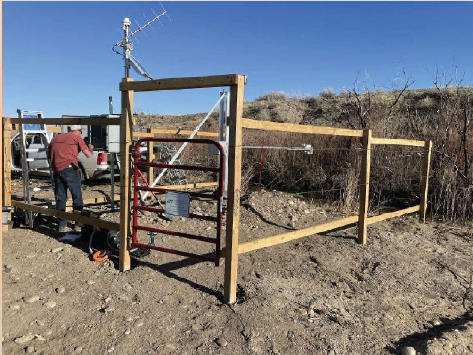
Radar installation, Purgatoire River at Fisher's Crossing Photo by Joey Talbott
