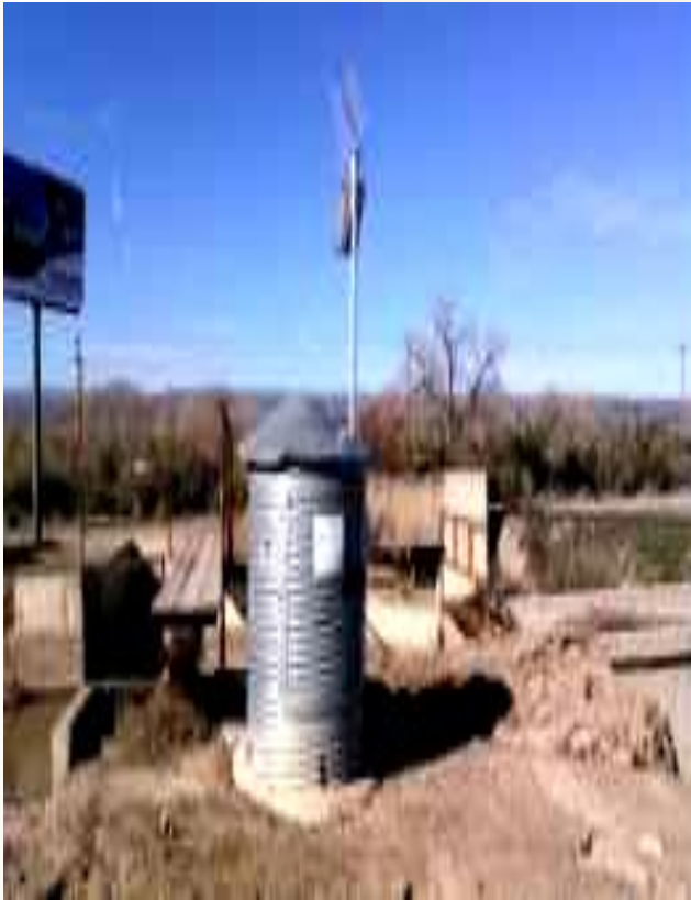
New Satellite Monitoring System on the Selig Canal
