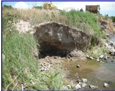
Empire Dam slope erosion
