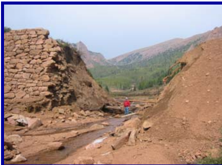
Failure of Gillett Reservoir Dam near Gillett, CO in Teller County, Division 2
