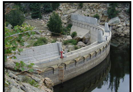
Tarryall Dam — Cracks found in the upstream face of the right gravity section of Tarryall Dam resulted in the lake being drained in response to a concern for the structural stability of the dam. The reservoir remains empty pending repairs.
