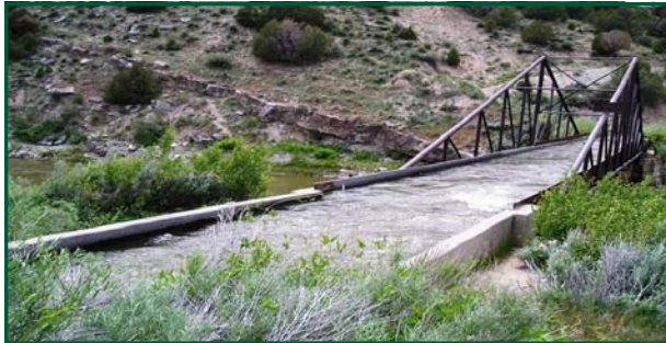
Maybell Canal diverts water from the Yampa River within the critical habitat reach
