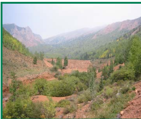
View of the breached dam observed on the September 7, 2006 site visit, from the access road below the dam.
