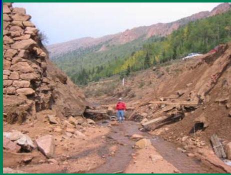
Looking east through the breached section from downstream to upstream. Note Water Commissioner for scale.
