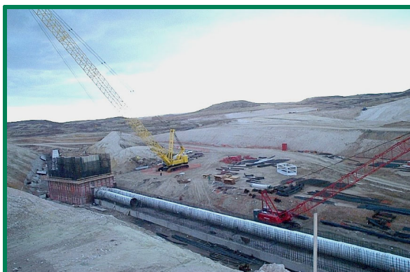
Construction of the output tower and the outlet conduit (comprised of two, 78-inch diameter steel pipes encased in reinforced concrete).
