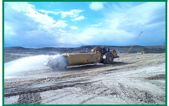
Clay soils are pre-treated with water before excavation. A fleet of scrapers move the treated clay and places it in the dam's core.
