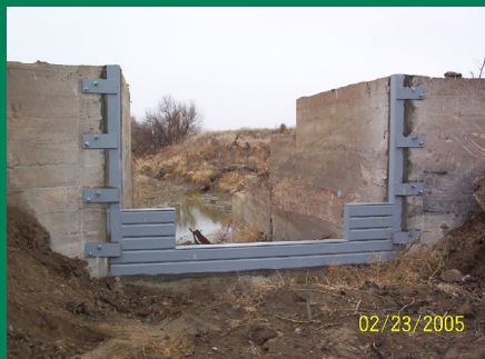
Two-staged weir retrofitted into an existing control on the inlet to Holbrook Reservoir to provide a means of measurement of reservoir deliveries by ROY participants or Holbrook Mutual Irrigation Company.
