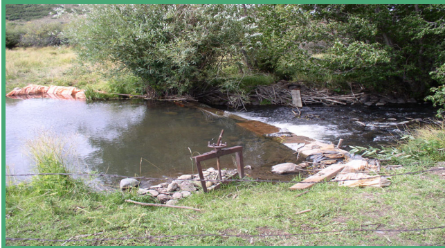
Before construction — Ira Van Camp headgate in the foreground and the Bird Ditch on opposite sides of the creek with plastic tarp used as headgate. Cement blocks are in the creek.
