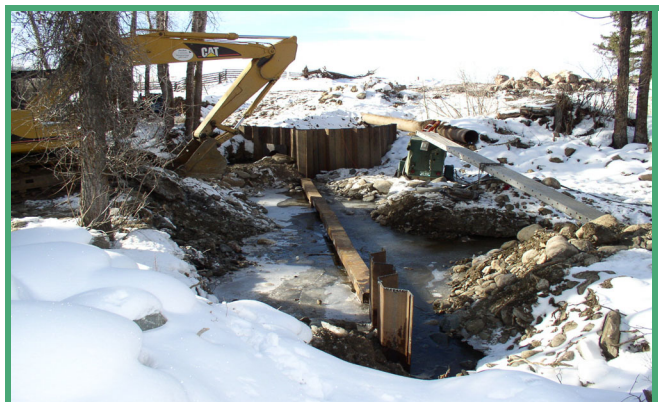
During construction of the new diversion dam and headgate for the Enterprise Ditch.
