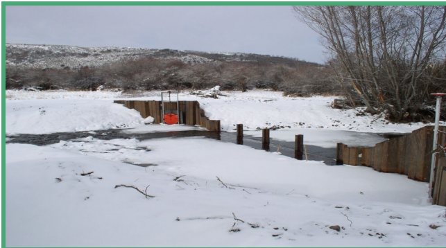
After construction — new diversion and headgates. Boards will be placed between steel uprights to create the diversion dam.
