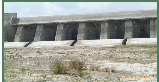
Reservoir Outlet Gates at Pueblo Reservoir
