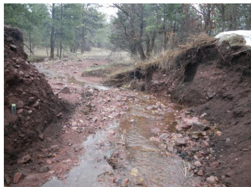
Illegal dam failure, Division 2
