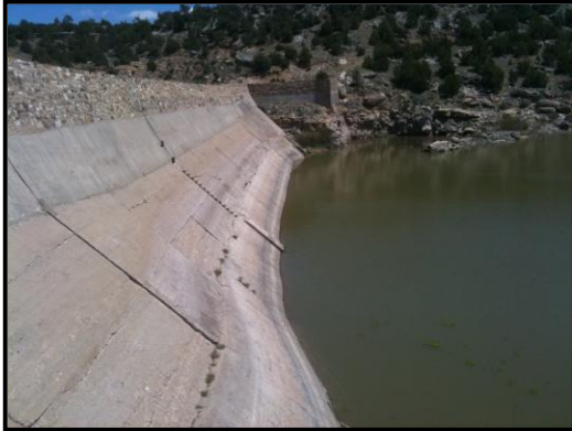
Cucharas Dam, Huerfano County High Hazard
