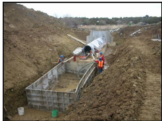
Martin Dam, Huerfano County High Hazard
