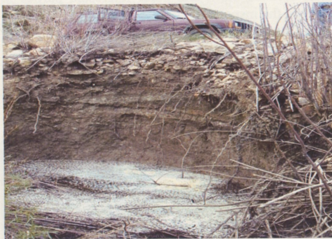
McElroy Dam Sinkhole Grand County Division 5, Low Hazard
