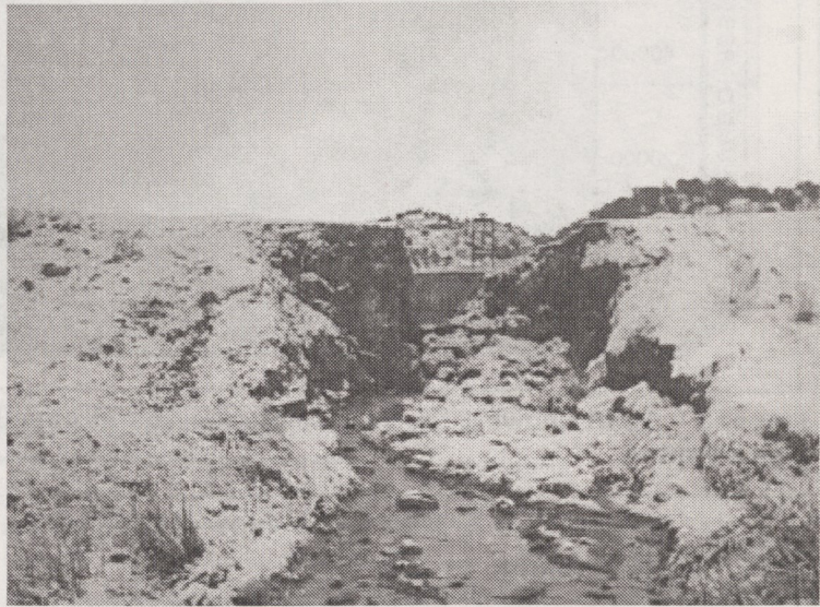
Sierra Pinyon Dam after being breached by a piping failure.
